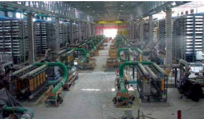
Figure 1: The Torrevieja 200,000 m³/day SWRO plant using ZERON 100 SDSS. Courtesy, Rolled Alloys.
